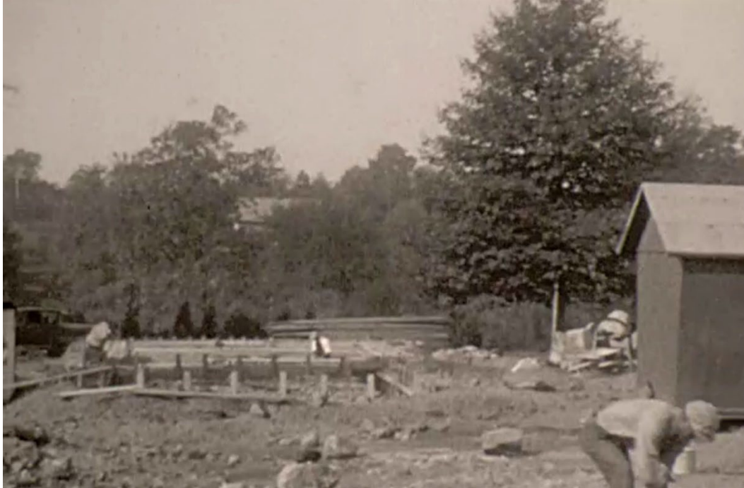
Figure 4.16a Circa 1929 still image capture from a Mather family home video. The newly constructed foundation of the barn appears in the midground of the image. A small outbuilding, apparently lifted from its foundation, is seen to the right. A vehicle on the left side of the image indicates the entry drive. Beyond the truck, a line of trees and shrubs marks the west edge of the drive. Courtesy McPherson-Nickerson family.
