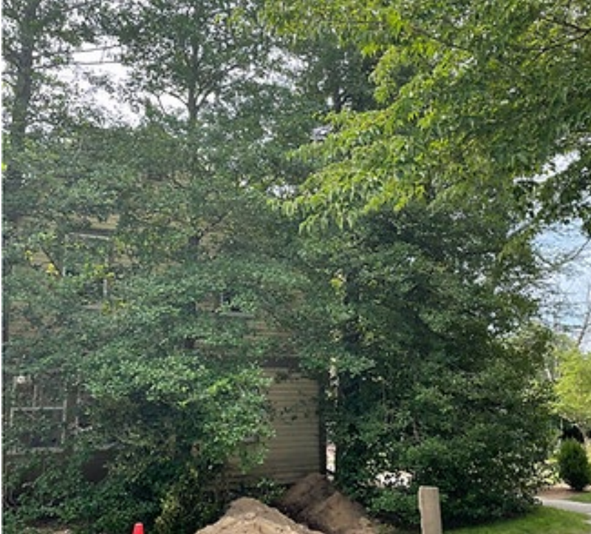
Figure 3.7a 2021 photograph of the east house façade, showing work underway to remove large trees near the building. Courtesy MHF.
